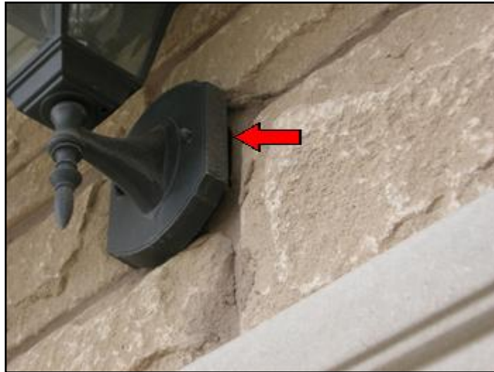
21. Gaps behind fixtures
