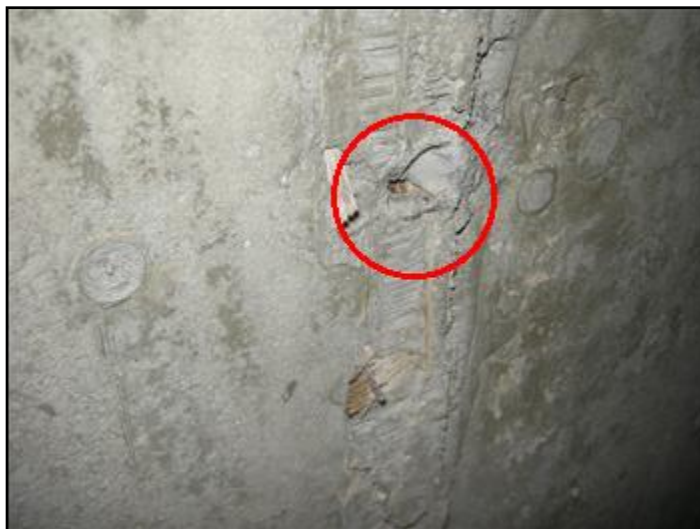
2. Tie-rod holes not sealed
