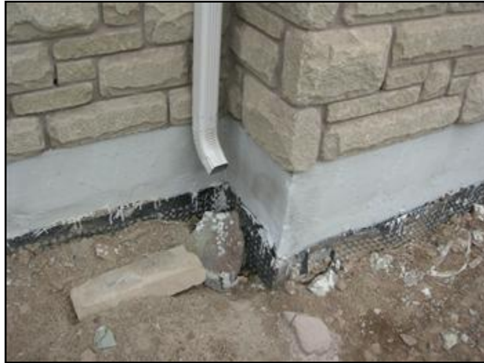
23. Incomplete work noted
