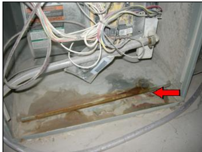
10. Leaky condensate line noted
