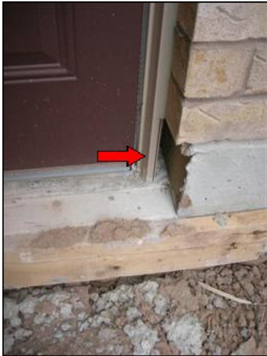
3. Gap at rear man-door to garage
