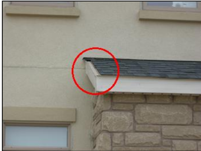
17. This condition on both sides
