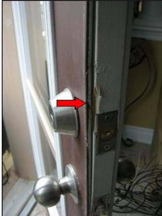
13. Damage at door
