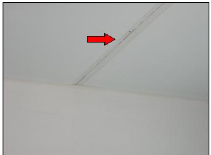
7. Area where drywall tape has fallen
